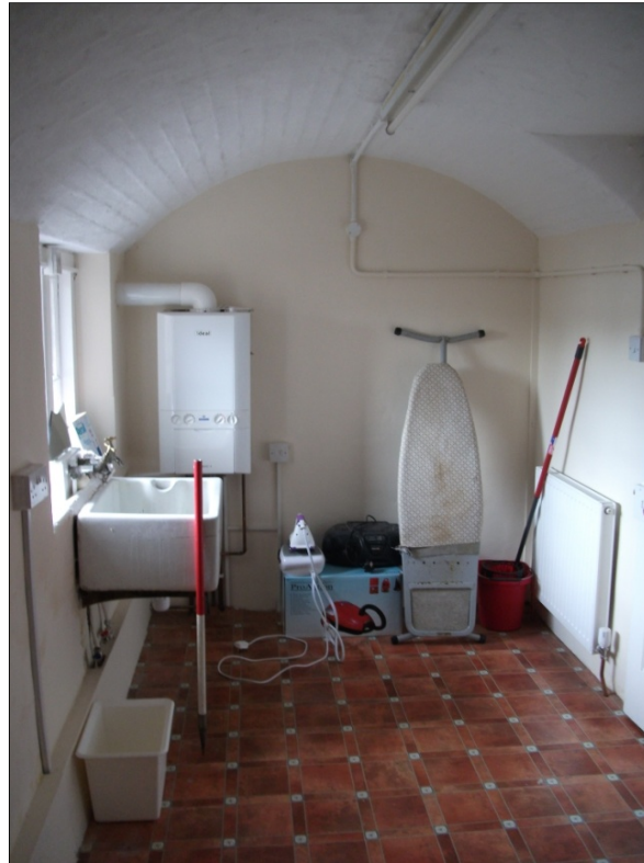
Fig 25: West wall of the Utility Room (G3) in the Old Bothy, looking W.
