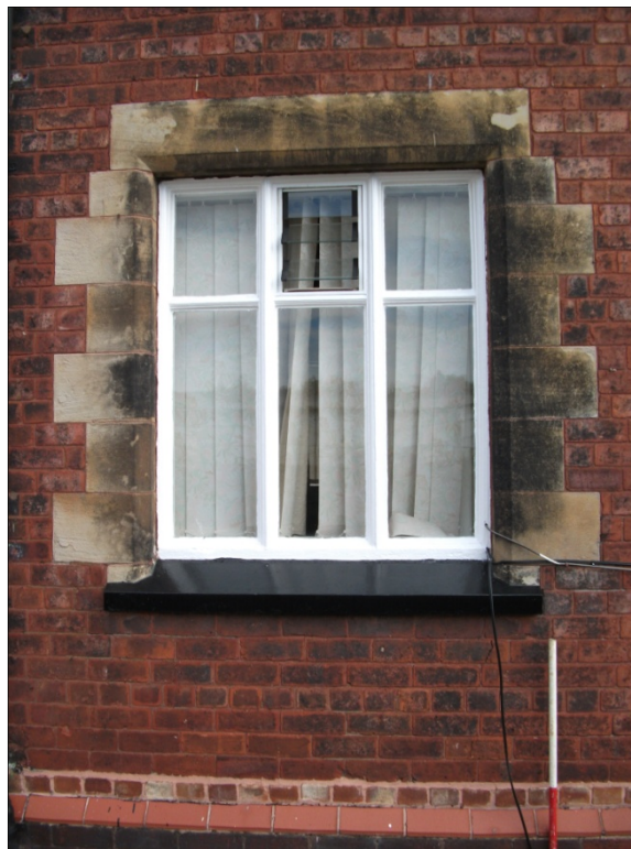
Fig 12: Ground floor window at western end of Bothy's southern elevation, looking N.
