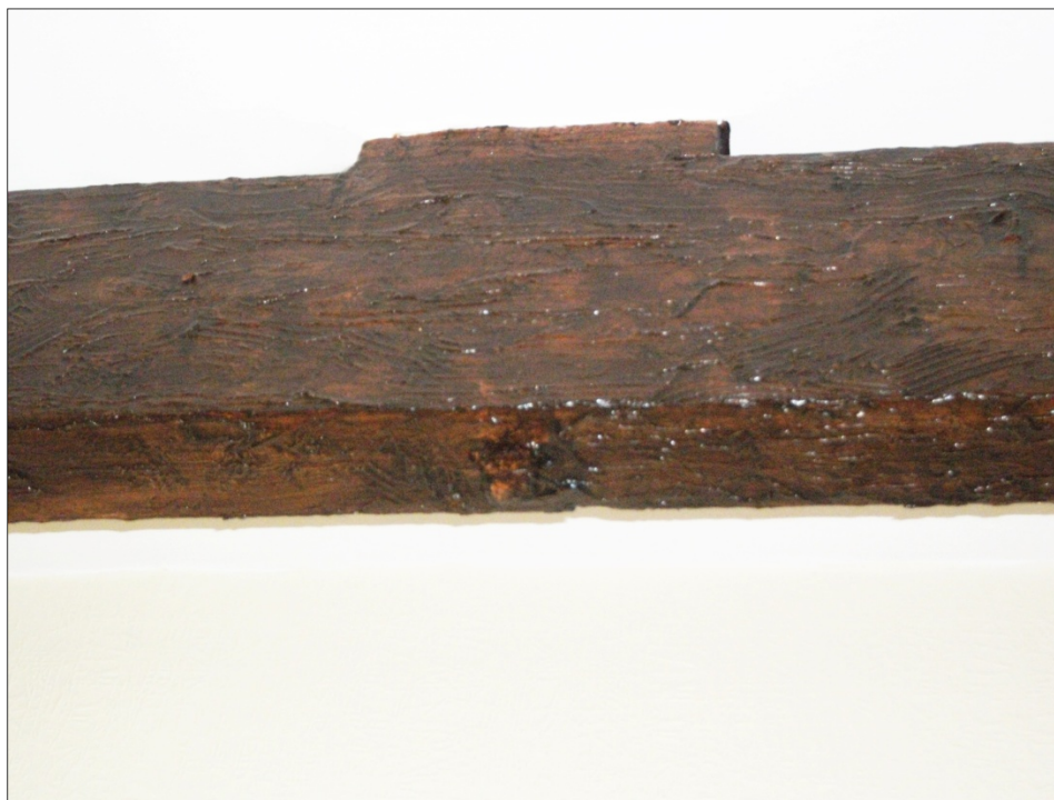
Fig 40: Detail of King Post Truss exposed in ceiling of Bedroom 3 (F4), Looking W.
