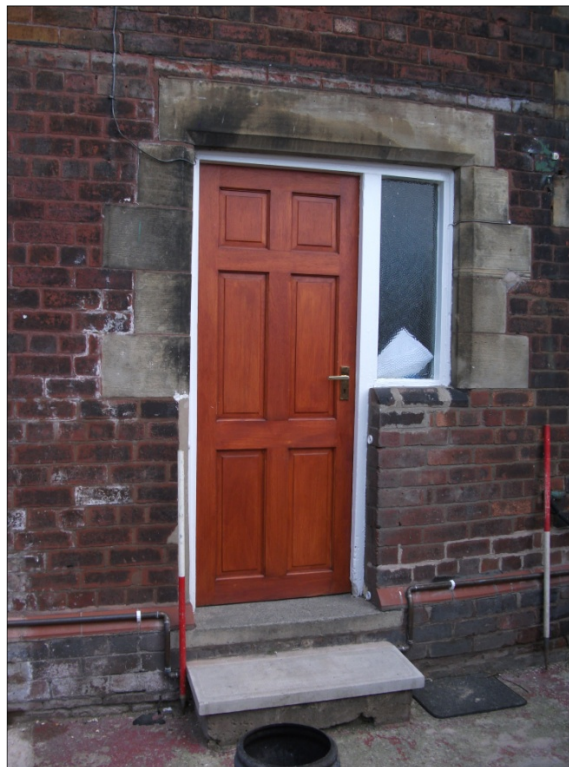
Fig 14: Former ground floor window, on south elevation which has been converted to a doorway, looking NE.
