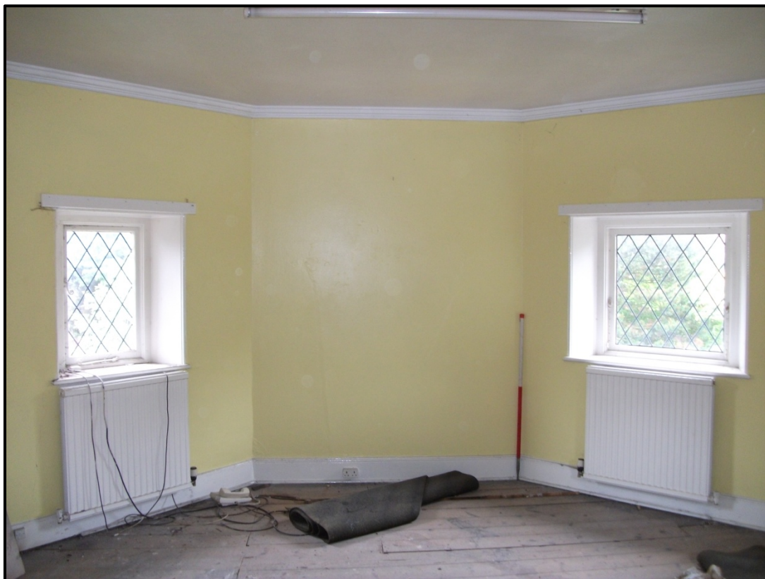
Figure 31 - View of the eastern walls of the Octagonal Bedroom (F3). Looking south-east
