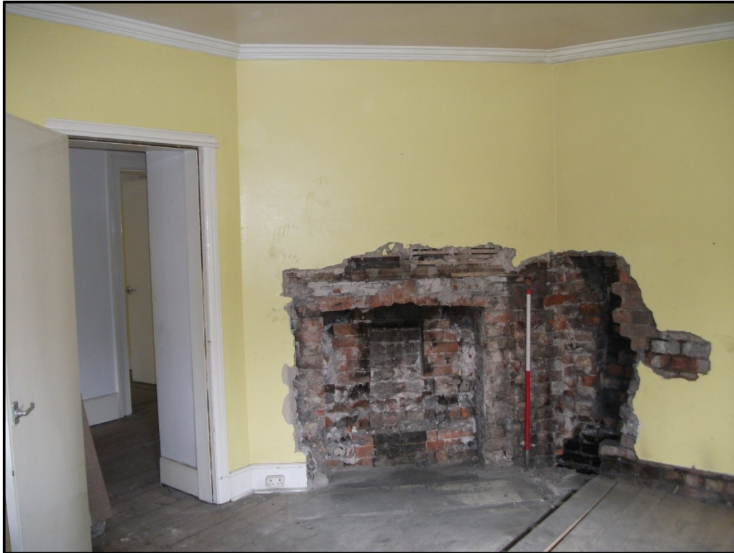
Figure 30 - View of the fireplace in the north-western wall of the Octagonal Bedroom (F3). Looking north west
