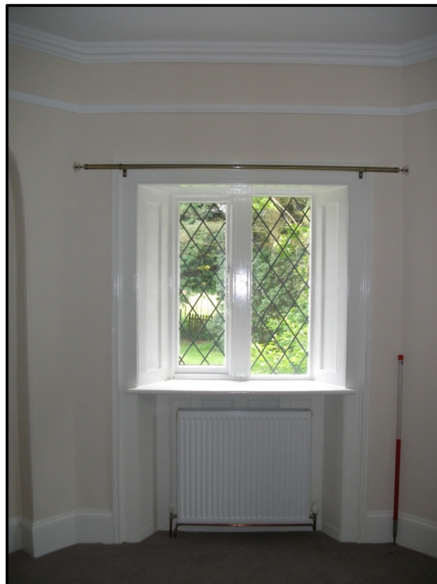
Figure 19 - Wood panelled window in the eastern wall of the Octagonal Sitting Room. Looking east
