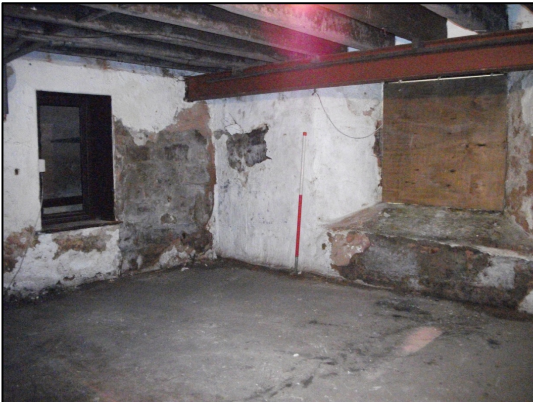
Figure 17 - View of the southern and eastern walls of the Cellars southern room. Looking south-east
