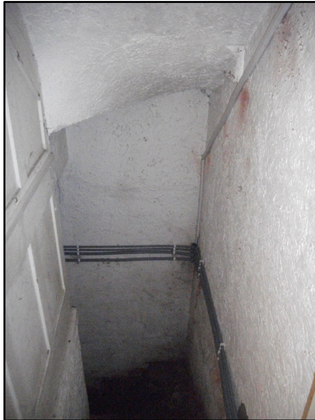
Figure 14 - A view of the entrance into the cellar from the ground floor hallway. Looking north-west
