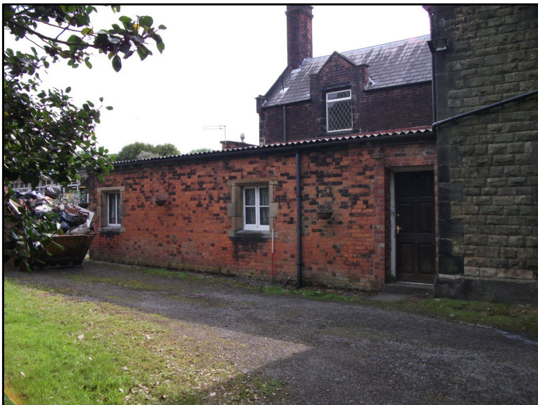
Figure 11 – View of the north end of the Garden Cottage, western elevation. Looking north-east
