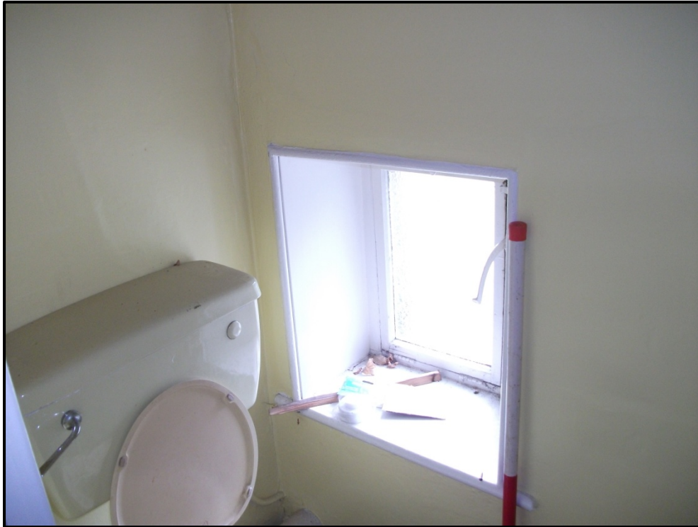
Figure 28 - Detail of window on the south wall of the first floor WC (F1). Looking south-west
