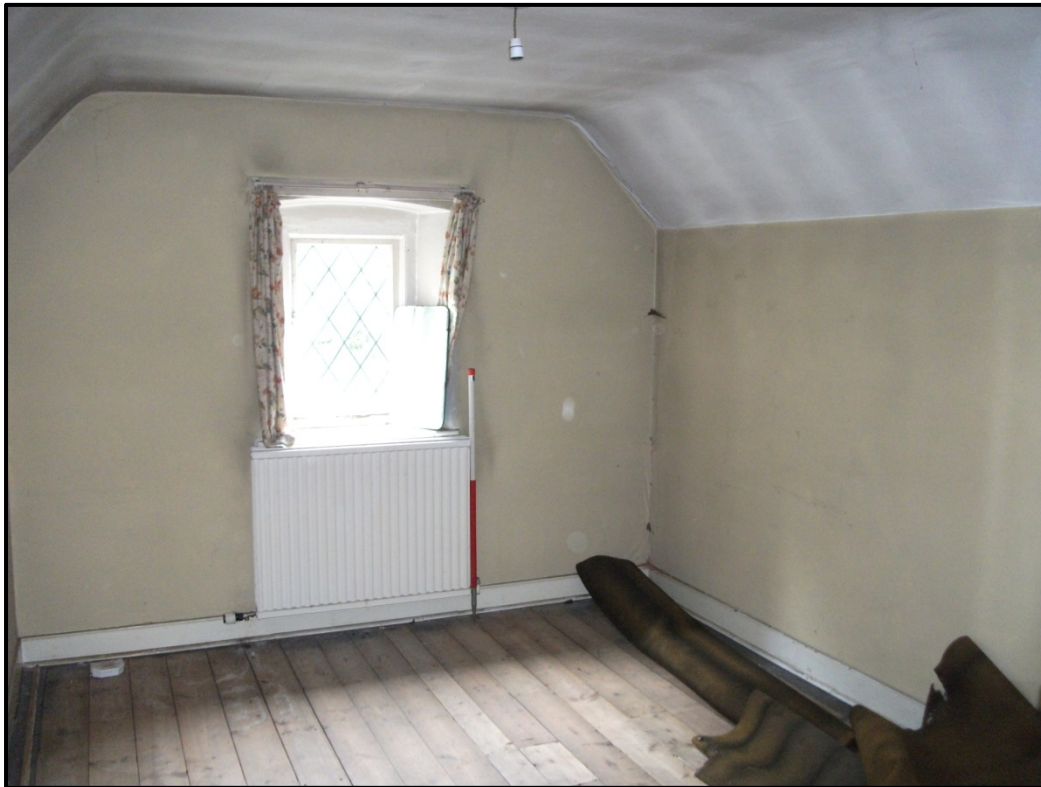
Figure 34 - View of western and northern walls of the Central Bedroom (F5). Looking north-west
