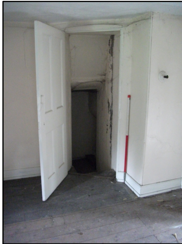
Figure 40 - View of the doorway in the north-western wall of the Octagonal Attic Bedroom (A1). Looking north west
