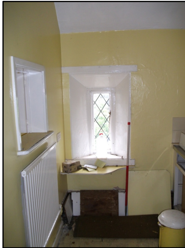
Figure 38 - Detail of window and serving hatch on the eastern and northern walls of the Kitchenette (F9). Looking east
