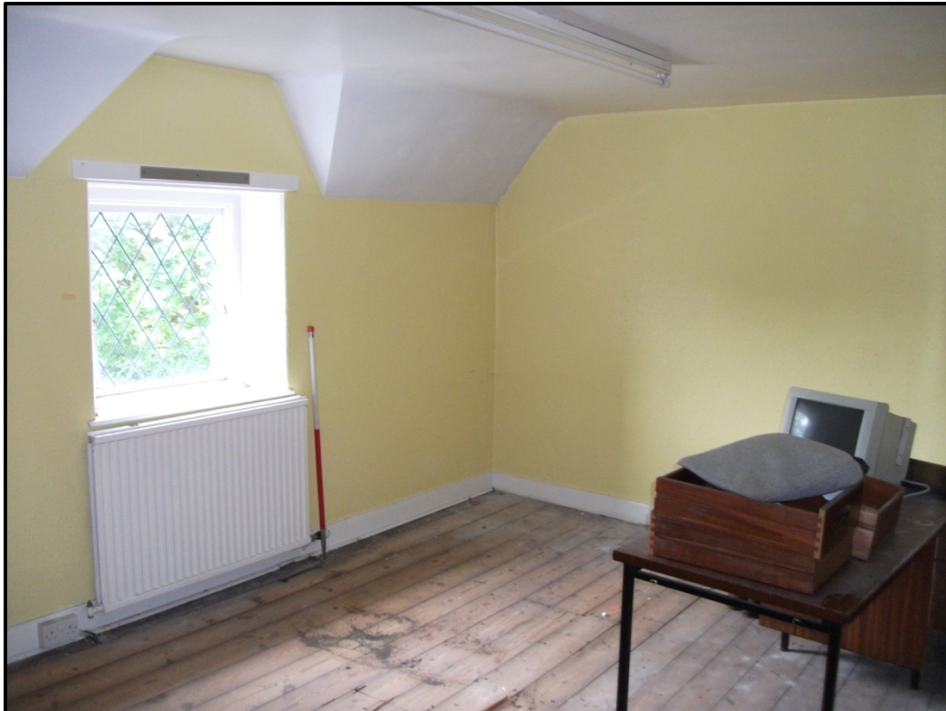
Figure 32 – View of the southern and western walls of the South Bedroom (F4). Looking south west
