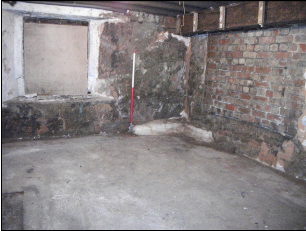
Figure 16 - View of the northern & western walls of the Cellars north room. Looking north-west
