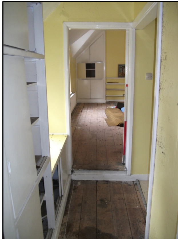
Figure 37 - View of first floor, Rear Hallway (F8) leading to the North Bedroom (F100) and Kitchenette (F9). Looking north
