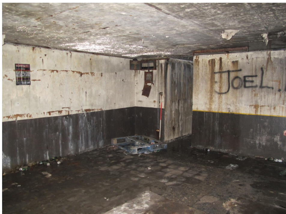
Figure 32: General shot of room F2 showing the access to room F3 along the northern wall and a series of possible fuse boxes in the northwest corner of the room. Looking northwest.
