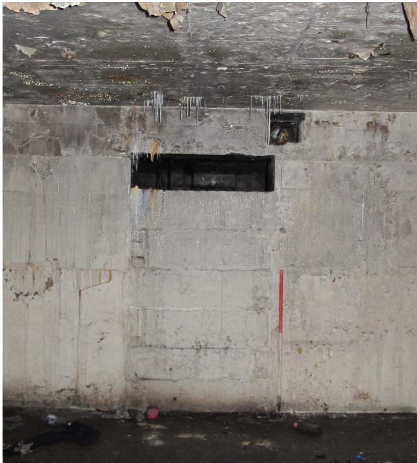
Figure 33: Detail of the most southerly blocked doorway along the east wall of room F2. This doorway would have originally lead to a walkway or room that ran around the top of the main operations room G4. Looking east.
