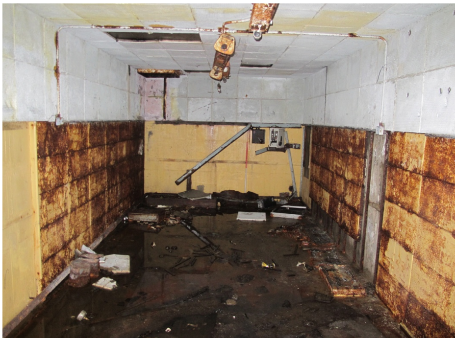
Figure 10: General shot of southwest radio control room G2 with sound proofing tiles covering the walls and ceiling. Looking west.
