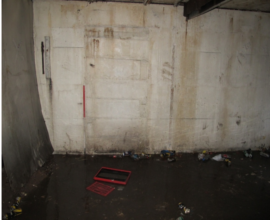
Figure 43: Detail of one of two blocked doorways located along the west wall of room F7. The doorway would have originally provided access to a walkway or room that ran around the top of the main operations room G4. Looking west.
