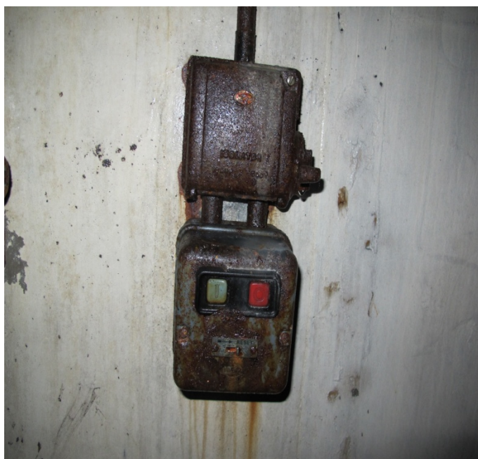
Figure 30: Detail of a power control system mounted on to the south facing wall of room F1. Looking north.
