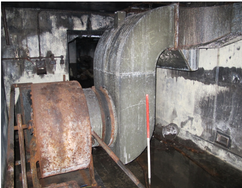
Figure 24: Shot of the air ventilation room G12, showing the central air handling unit for the building. Looking west.
