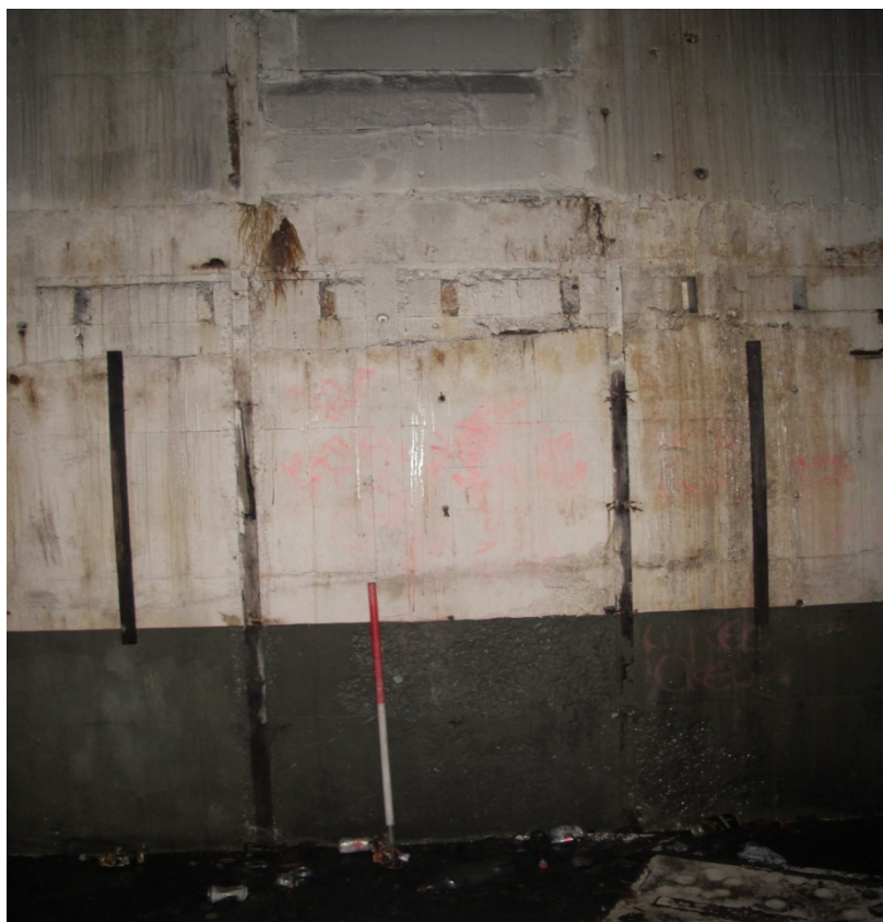
Figure 13: Detail of fixings for possible shelving on the east facing wall of the main operations room G4. Looking west.
