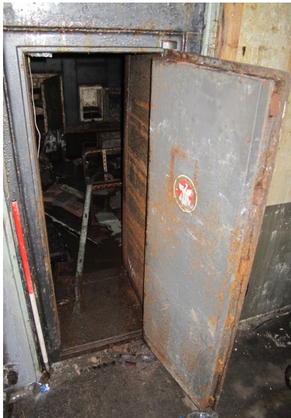
Figure 19: Detail of the main door into to the safe room G9. Note the reinforced steel surround and double thickness iron door. Looking south.
