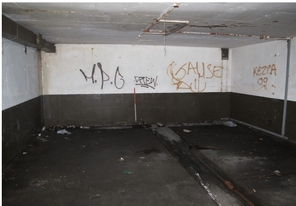
Figure 15: General shot of room G7, showing the floor with a 'T-shaped' wooden in-lay. Looking west.
