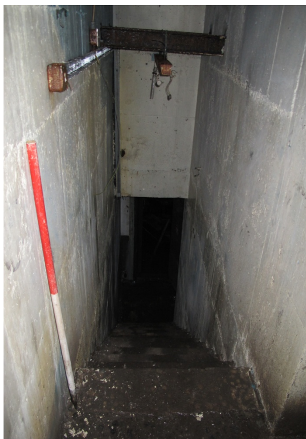
Figure 28: Shot taken of north eastern staircase S4, looking down the staircase from toilet room F6. Looking south.
