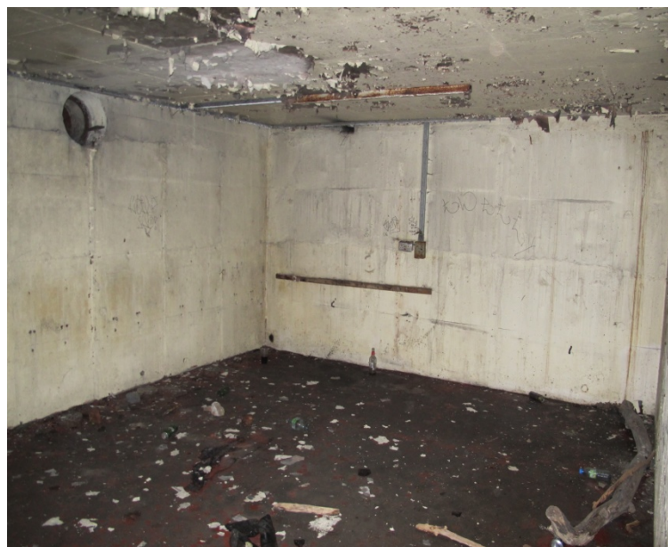
Figure 34: General shot of room F3 showing light switch on the north wall and an open air vent cut through the west wall. Looking north.
