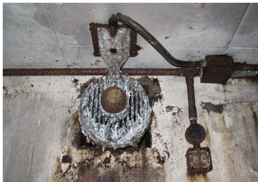
Figure 40: Detail of a corroded fan located on the east-west aligned partition wall in room F6. Looking north.
