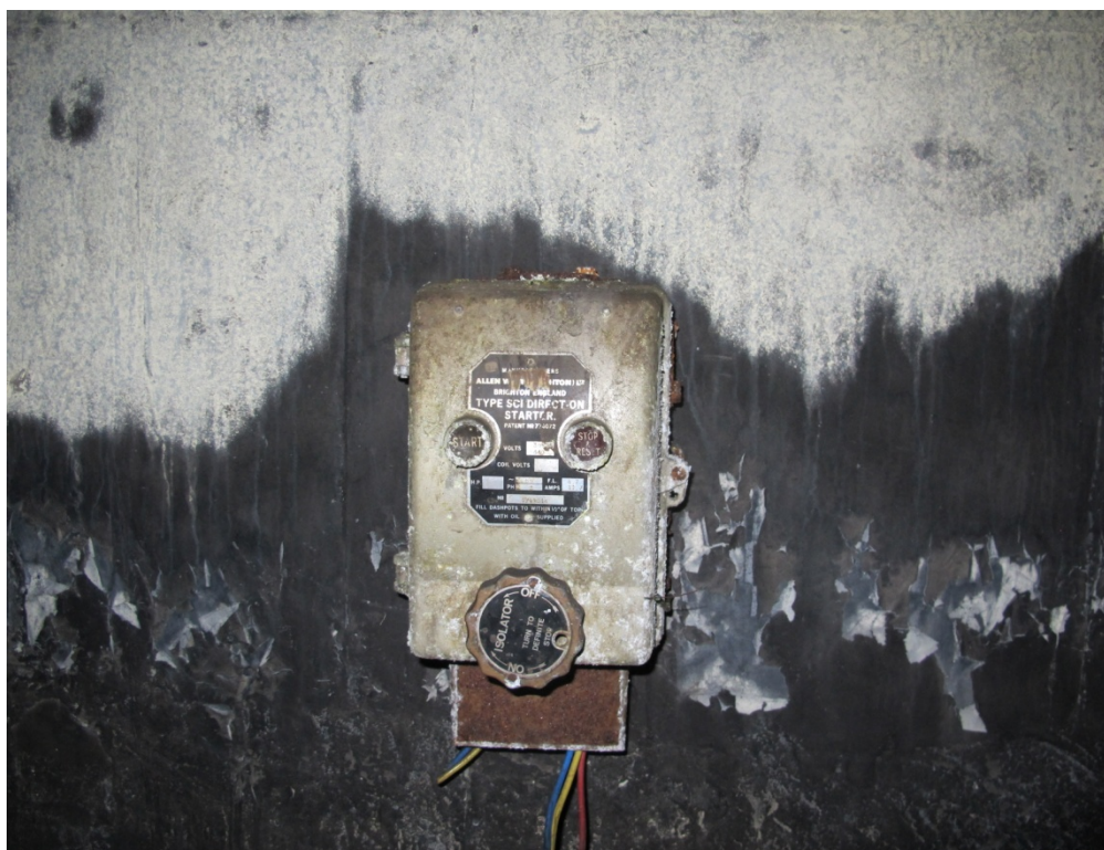
Figure 25: Detail of wall mounted control device for the ventilation unit in room G12. The device was fixed to the south facing wall of the room.
