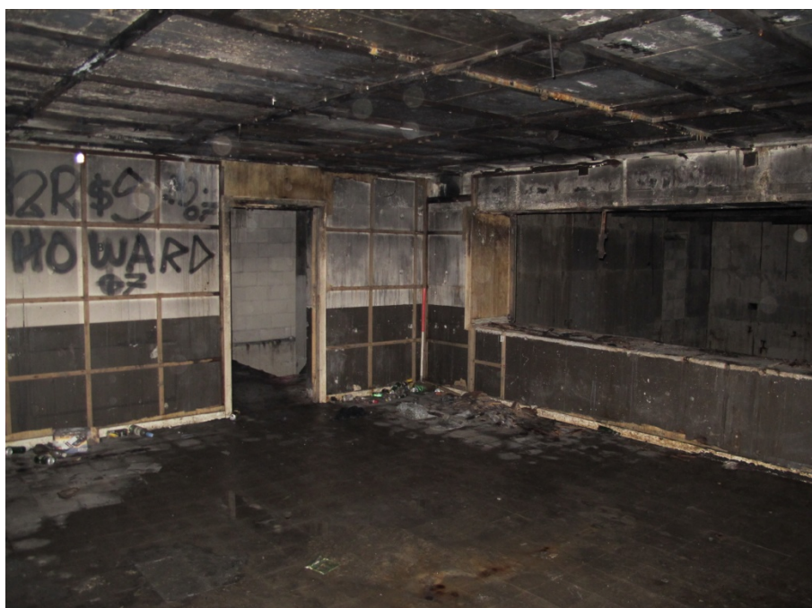
Figure 38: General shot of the viewing gallery room F5 showing the eastern doorway and the viewing window that looks down on to the main operation room G4. The walls and ceiling were found to be covered in wooden framing, a likely mounting for wooden panels. Looking southeast.
