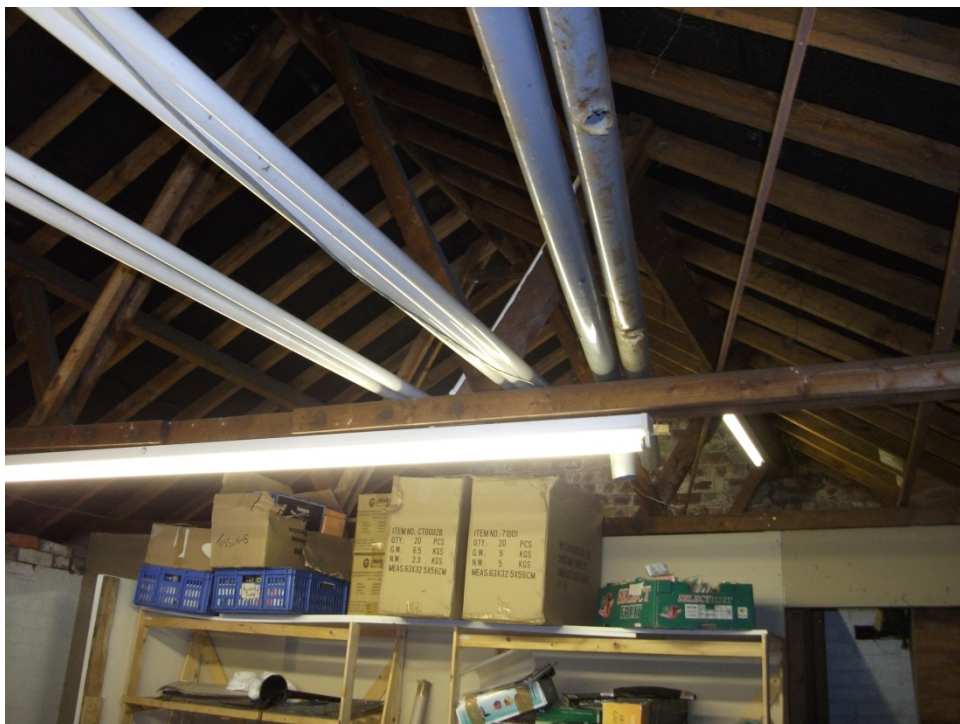
Fig. 16 - View of roof timbers exposed within the first floor of the barn. Looking N
