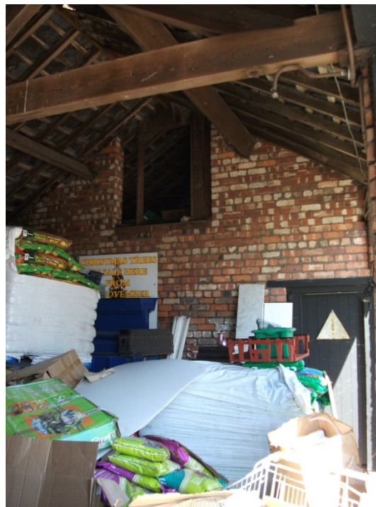
Fig. 10- View of the partition wall dividing the southern and northern bays of the Stables. Looking N
