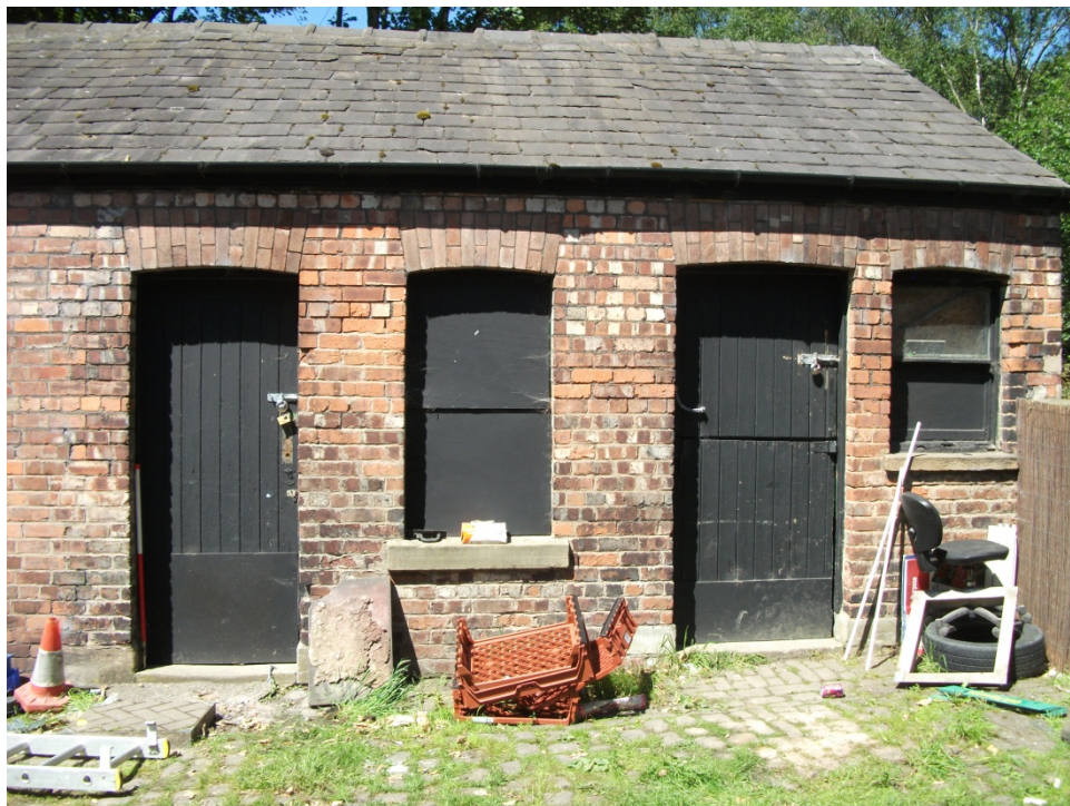
Fig 12 - View of the north end of the Stables eastern elevation. Looking W
